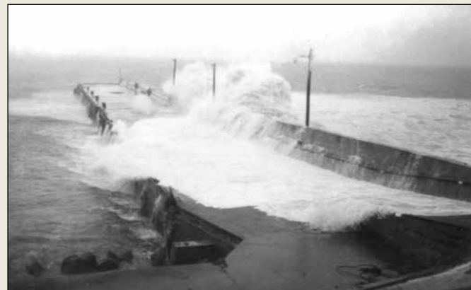
Figure 1.4. Overtopping during a storm at the pier of Hofsós before construction of the berm breakwater.
