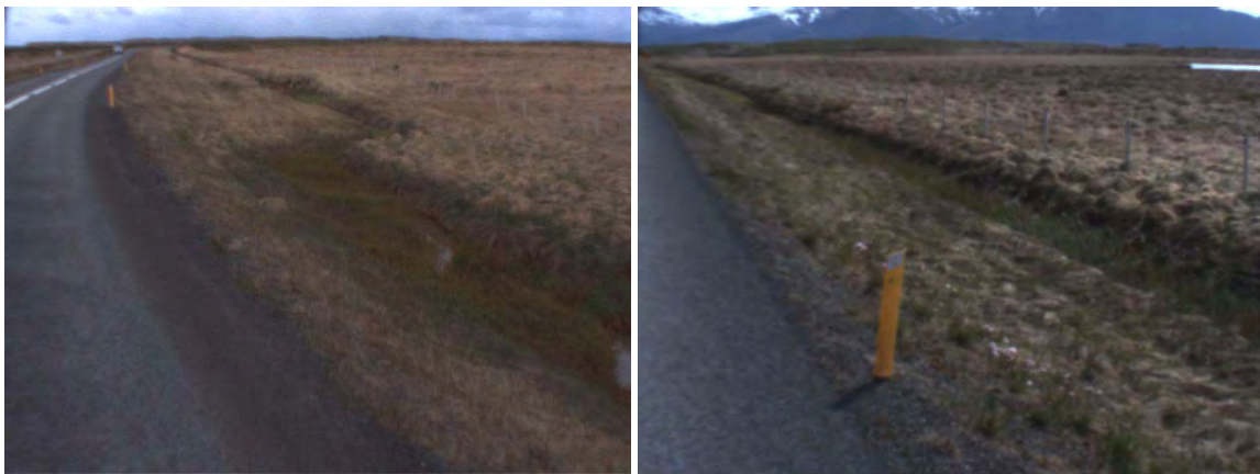
Figure 52: Water standing in the ditches (chainage left: 6760m, right: 7020m).
