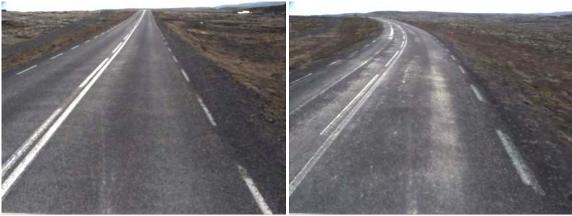
Figure 44: Dry terrain in the end part of the section (chainage 9900m (left), 11000m (right)).
