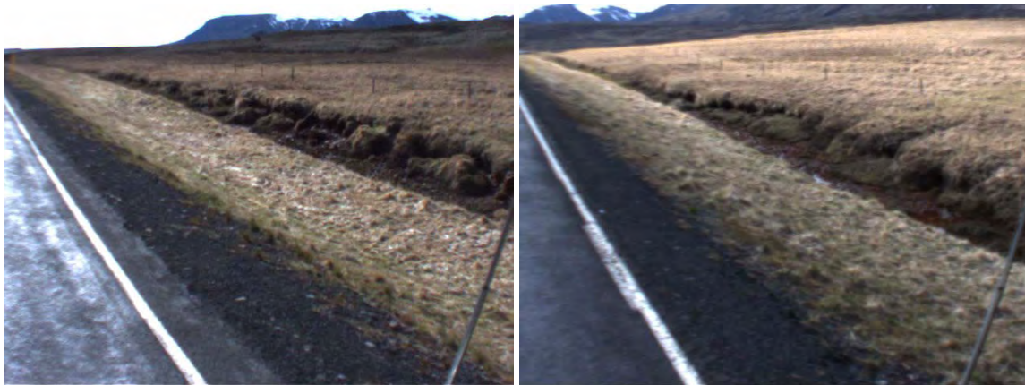
Figure 38: Unstable material was hindering water flow in the ditch (chainage 480m and 890m)
