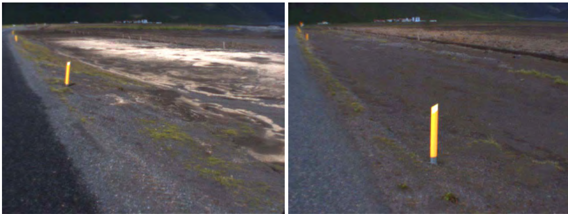
Figures 18: Volcanic ash from the eruption was still visible in the ditches (at chainages 130m and 480m)
