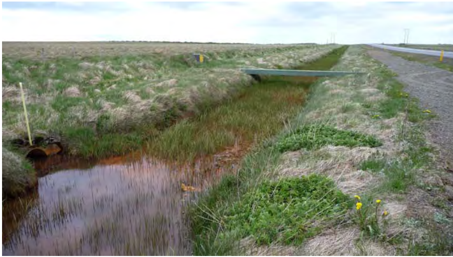
Figure 46: Ditch full of water and vegetation at chainage 4380m.
