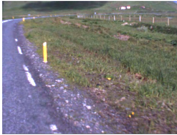
Figure 15: Minor drainage deficiencies on a curve. The ditch was placed far from the road behind the horse track (9480m).
