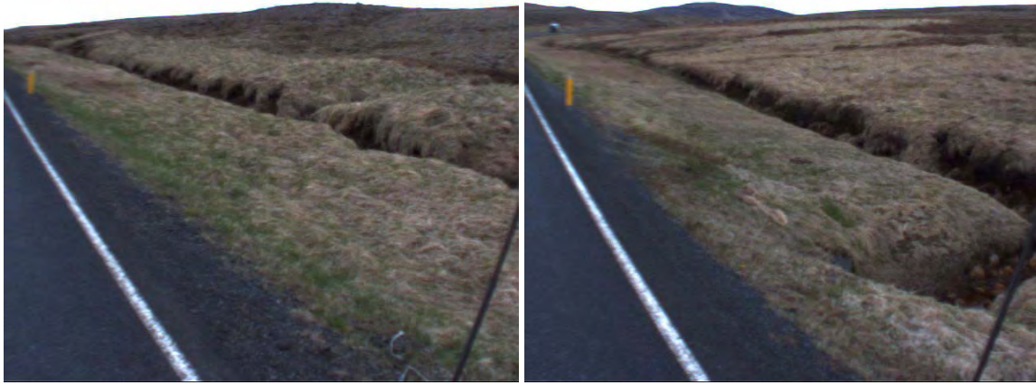
Figure 39: Collapsed ditch walls on the upper side of the road profile at 4690m and 5450m.
