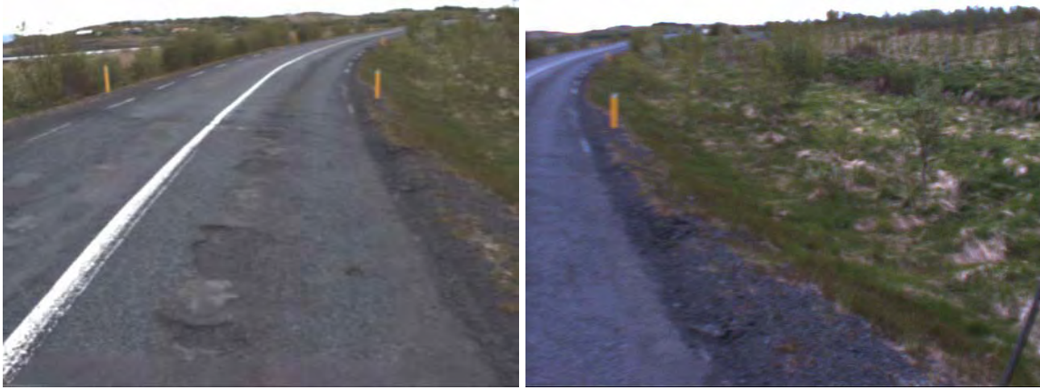
Figures 30: Inadequate drainage on the upper side of the side sloping profile. Left figure is the road camera view and the right figure is the ditch camera view, chainage 8810m.
