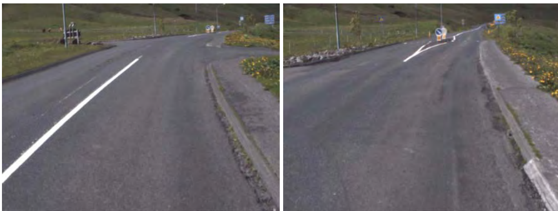
Figures 13: Footway kerb blocking water flow causing minor washout damages. Chainage on the left figure is from 10m, and on the right 30m.
