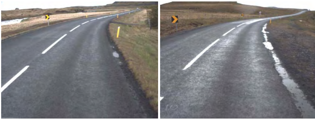
Figure 32: Verge preventing the water flow, chainage 6520m and 6760m.
