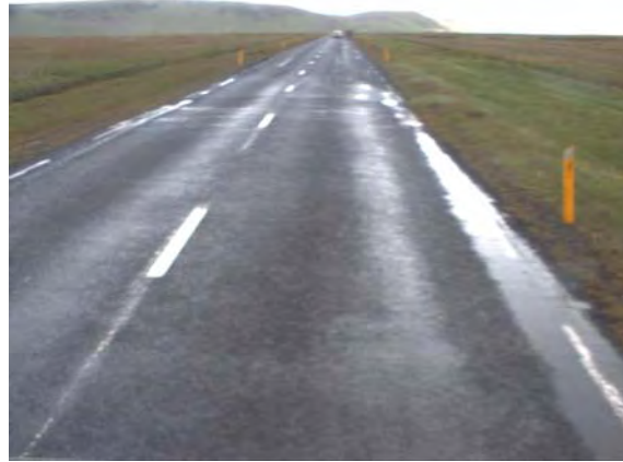
Figure 17: Verge is stopping the water on the edge of the pavement, chainage 3830m.
