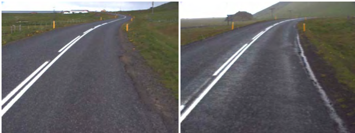
Figure 20: Shallow ditches and verge causing the water to infiltrate into the edge of the pavement (Chainage 2620m and 5700m).
