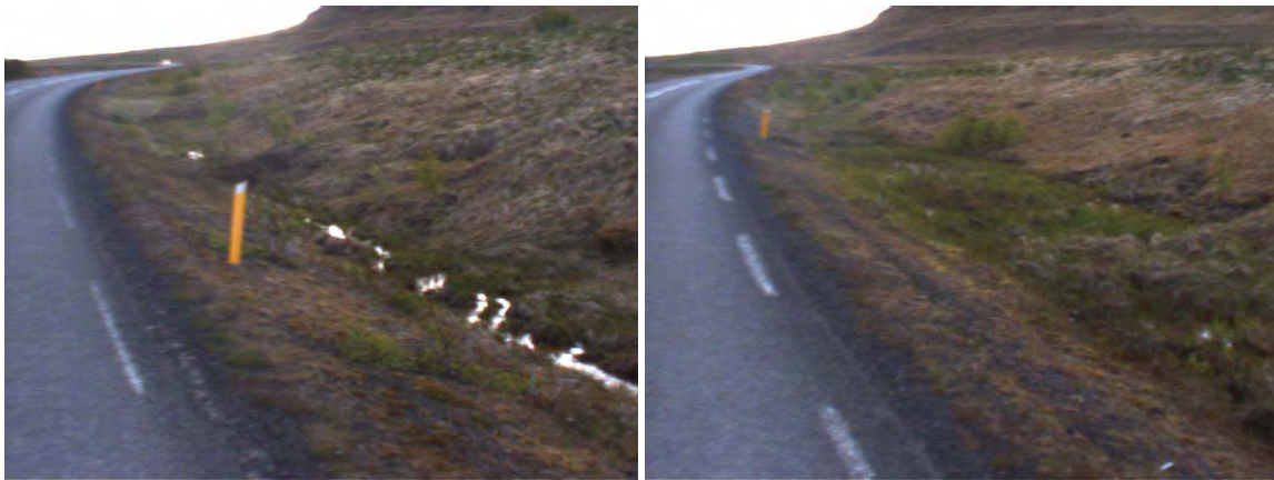
Figure 48: Unstable material on the bottom of ditch was hindering the water flow (chainage left: 7850m, right: 7890m).
