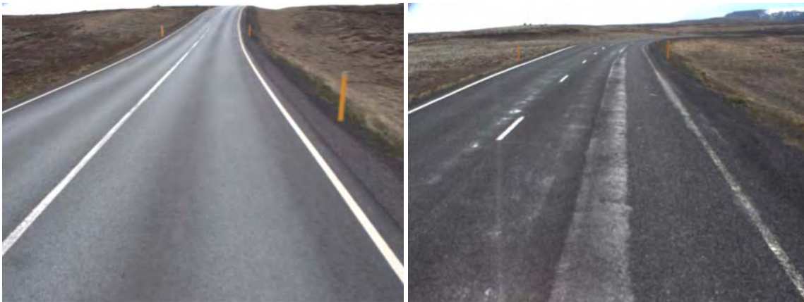
Figure 36: In road 36 section 07 the pavement condition varied but there were no drainage problems (chainage left 600m, right 2700m).
