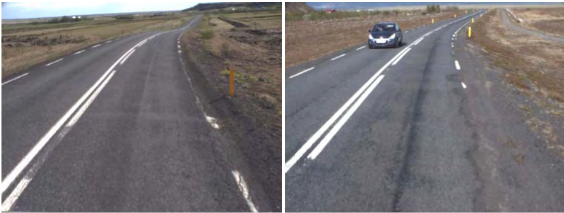
Figures 45: Verge was preventing the water flow from the pavement surface at times (chainage 4030m on the left, 11090m on the right).
