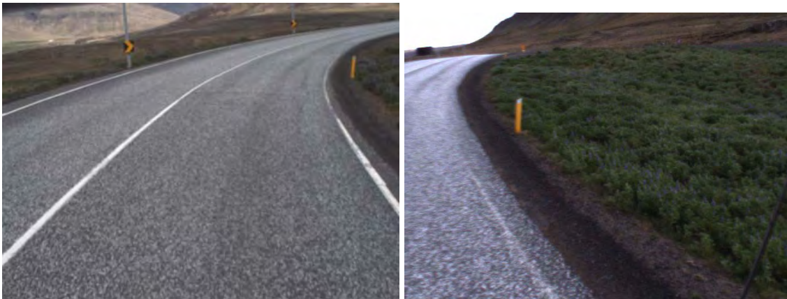
Figures 40: Insufficient drainage on the upper side of the steep side slope at chainage 6900m. The left is the road camera video and the right is the ditch camera video.
