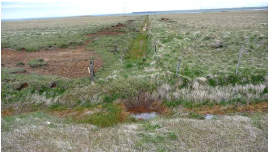
Figure 47: Blocked outlet ditch at chainage 4370m
