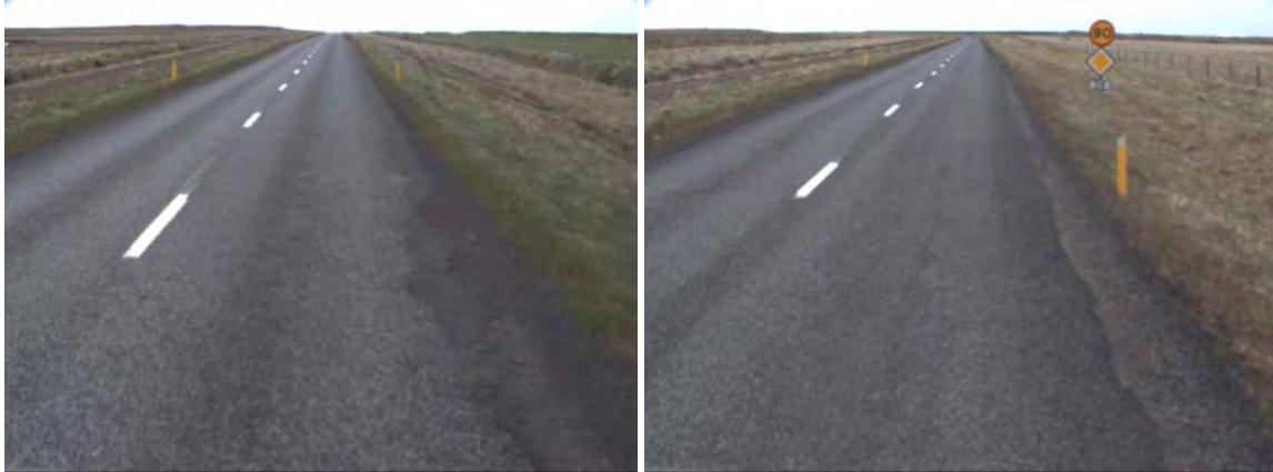
Figure 23: Verge hindering the water flow from the pavement surface (chainage 2850m, 3920m).
