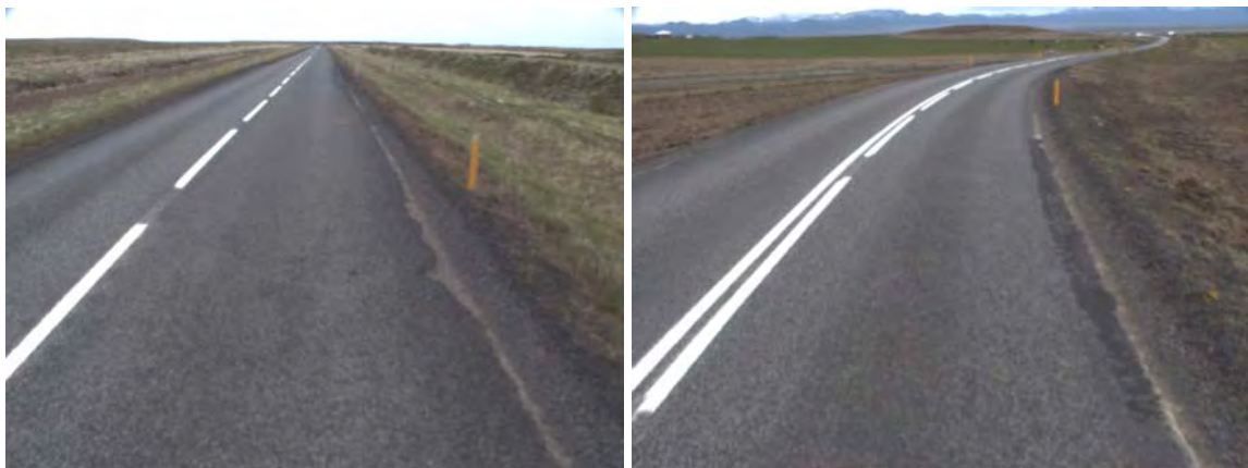
Figure 24: Problematic verge at chainage 4270m and 8830m.
