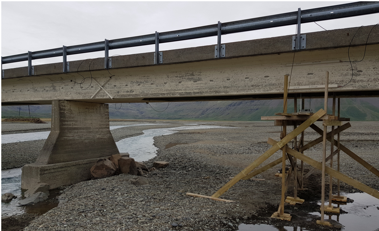
Figure 2.2: The OSMOS strain sensors installed on the girder and the LVDT differential displacement sensors on a timber platform.
